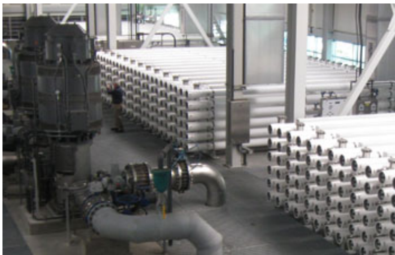
Figure 8 Industrial SWCA RO plant
