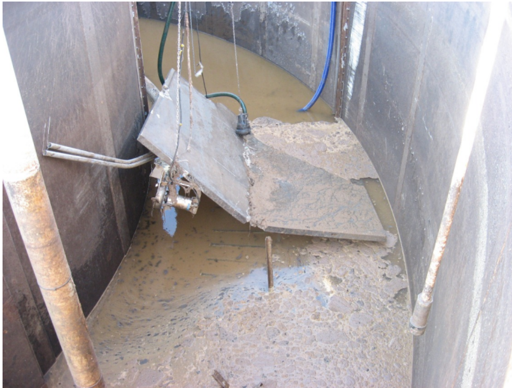
Photograph 2: Broken Bioreactor Panels - Pines Wastewater Treatment Plant 4 Sept 2010
