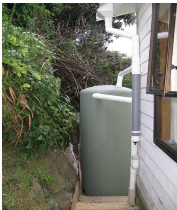
Figure 4: A 1,000 litre rainwater tank with screened rainhead and first flush diverter installed at dwelling in Paekakariki
