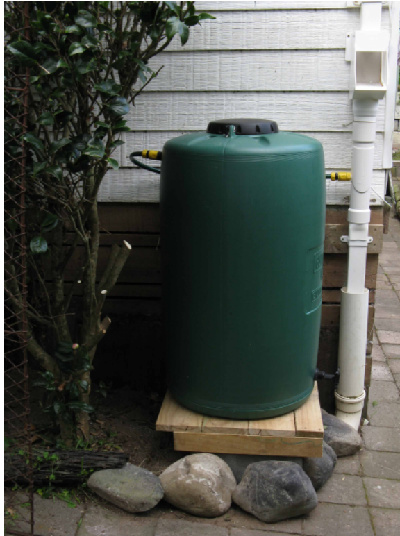
Figure 2: 250 litre rain barrel connected to down pipe via water collectors/diverter
