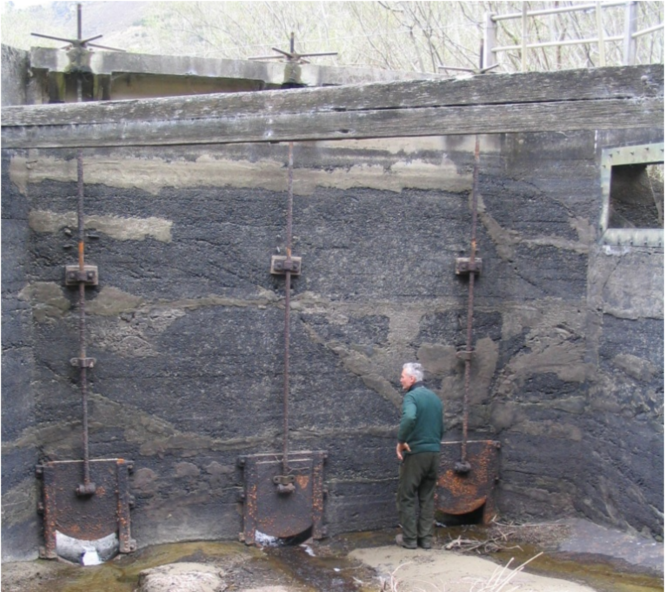
Photograph 2: De-silter at the outlet of Tunnel No. 1 of the Manuherikia Irrigation Scheme
