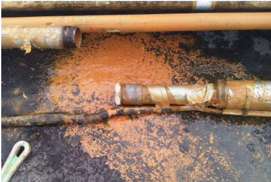
Photograph 3: Iron flocculation encountered when disconnecting Pak 'n Save bore pump
