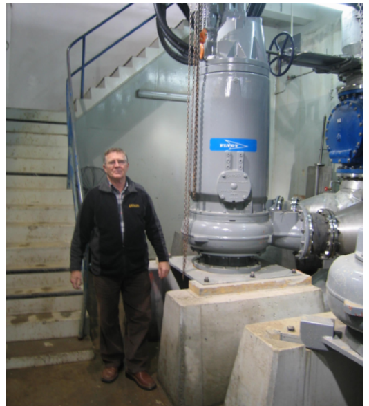
Figure 5: New 250kW Okara Park sewage pumps
