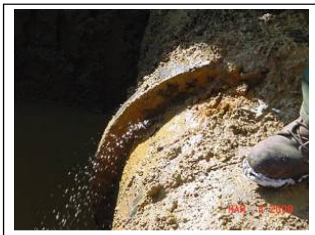
Figure 5. Small Leak in 900mm Pipe
