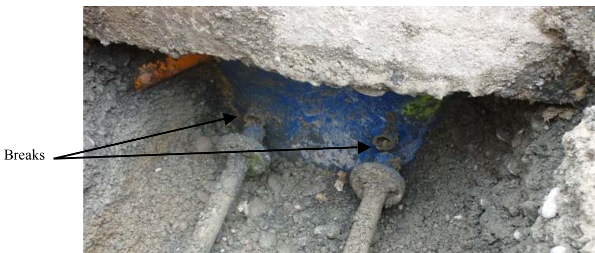
Photograph 13: Birchgrove Pump Station, Christchurch (PS97): Discharge pipes broke during 22 February 2011 earthquake at fibreglass spool just outside pump station wall.
