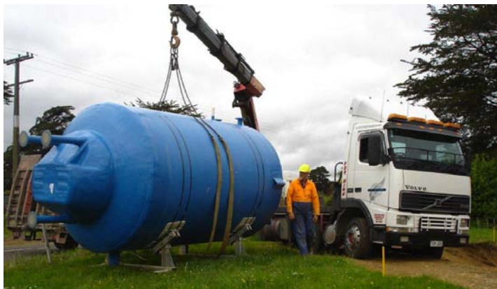
Photograph 7. Fibreglass pump stations are lightweight.
