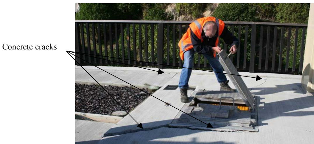
Photograph 15: Black Rock Pump Station, Lyttleton (PS625): Earthquakes cracked concrete surrounds.
