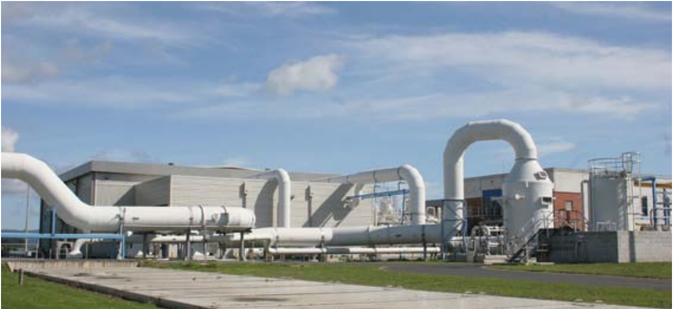
Photograph 1: Fibreglass Ducting, Fans, Scrubber, and Tank at Wastewater Treatment Plant
