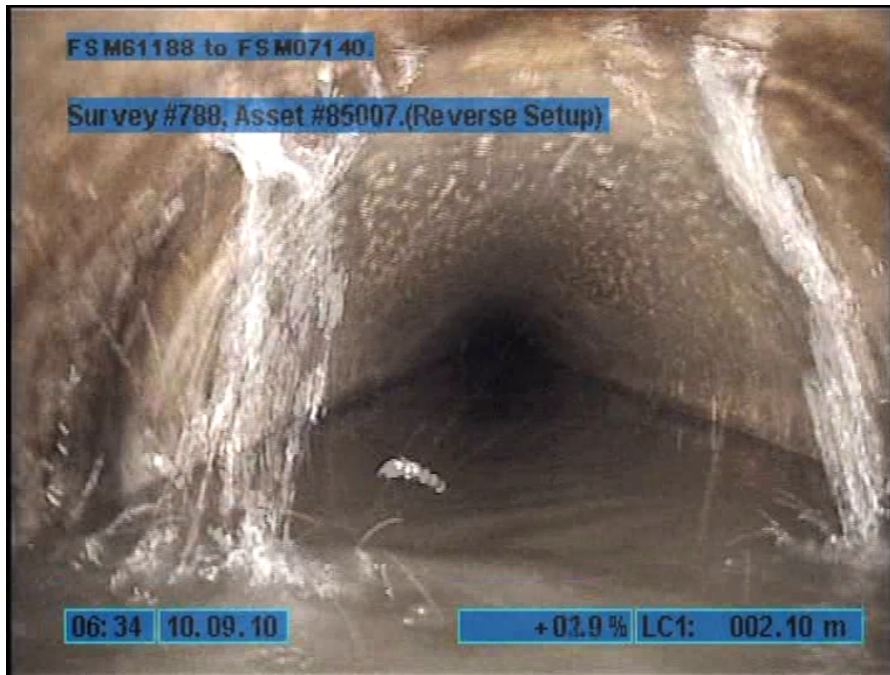
Photograph 3 – Still image from CCTV of the Marne Street line
