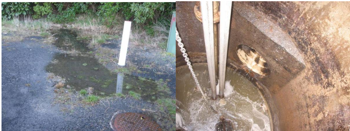
Photograph 11 and 12 – Upwelling of tidally influenced groundwater and saline infiltration in a wet well
