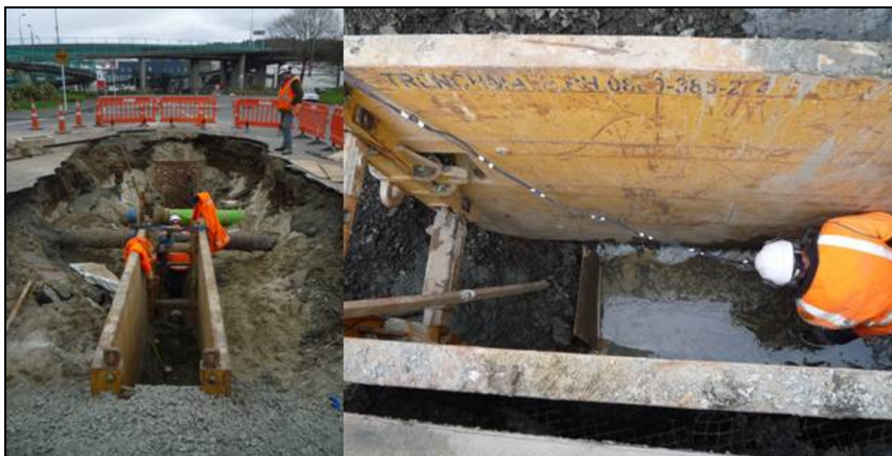
Photograph 7 and 8 – Photos of the Birch Street dig and lay of 80m of 225mm foul sewer
