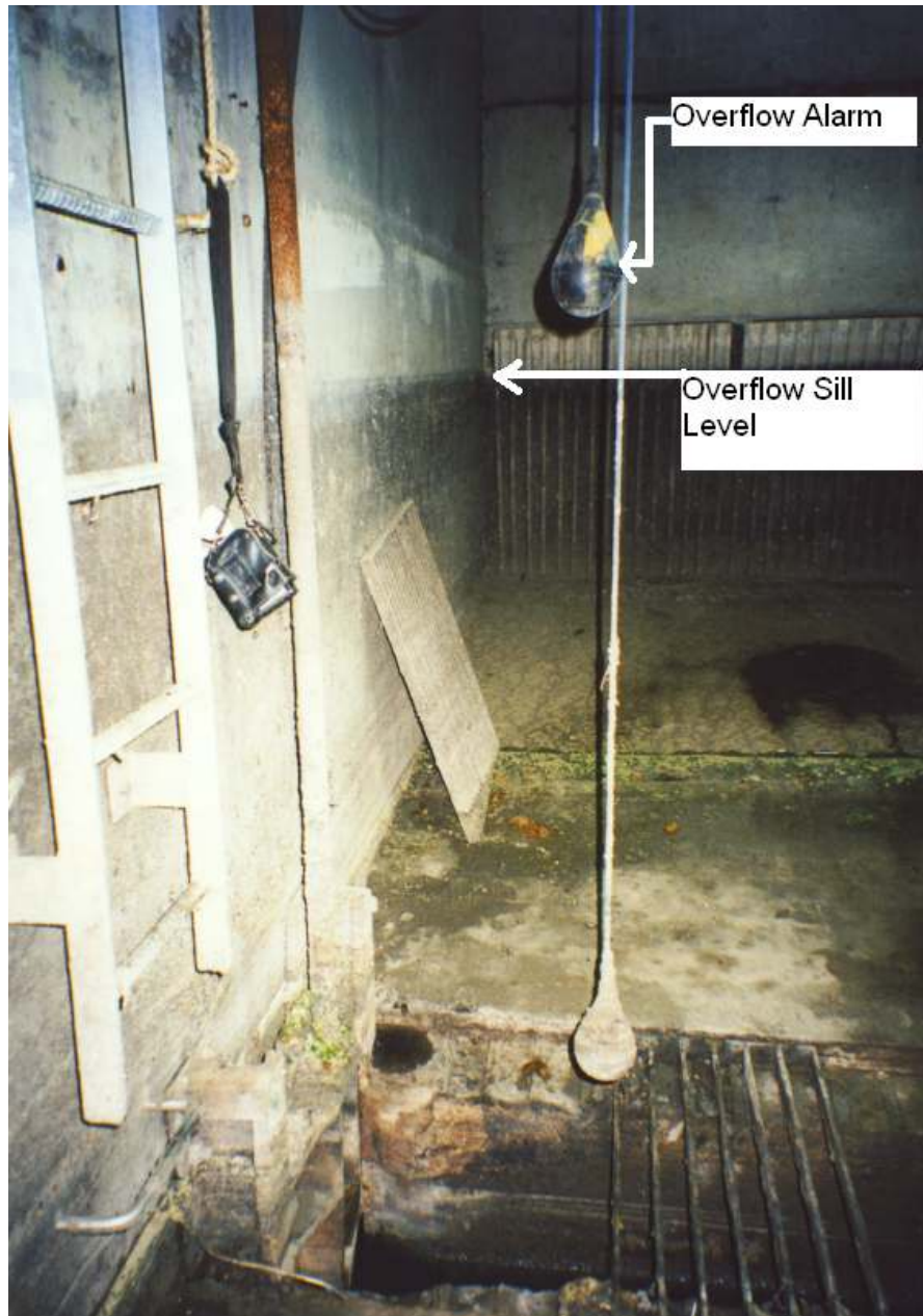
Photograph 2: Overflow Float Alarm Switch Above Overflow Sill Level
