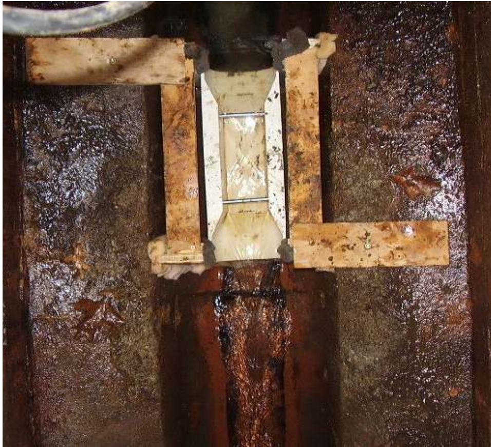
Photograph 1: Typical Flume Installation
