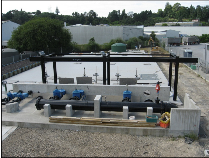
Photograph 1: The new Maleme Street Pump Station (control building not in view)
