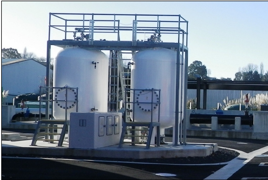
Photograph 8: Maleme Street Pump Station air vessels
