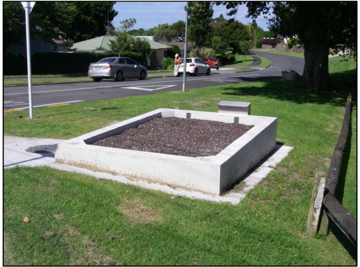
Photograph 5: Typical passive biofilter servicing an inverted siphon
