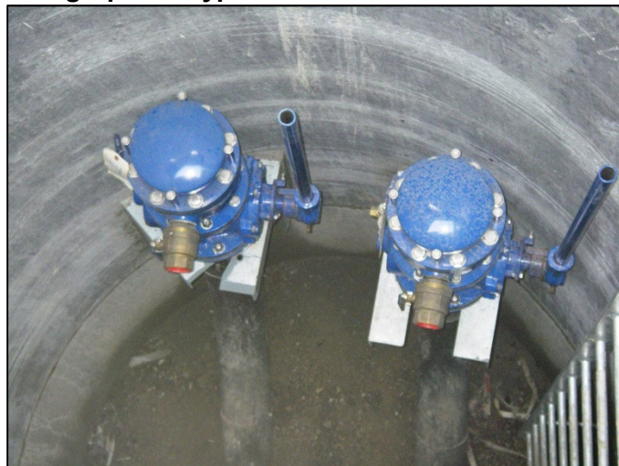
Photograph 6: Typical dual vacuum relief valves
