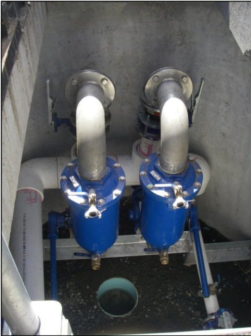
Photograph 4: Typical air valve system at the start of an inverted siphon
