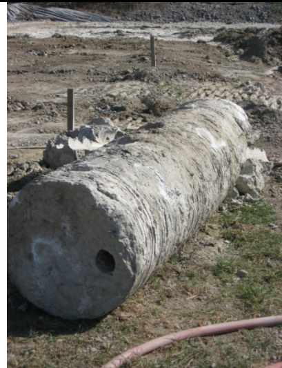
A deep soil mix column is removed and core for testing as part of the ground strengthening work, February 2008
