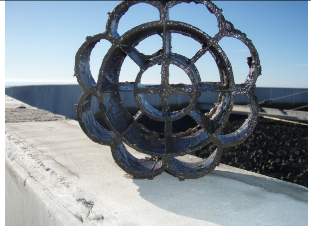
View of a Plastic Media (Petal) piece showing biomass growth (with 1 – 2mm covering) – taken from the full scale Biological Trickling Filter Plant
