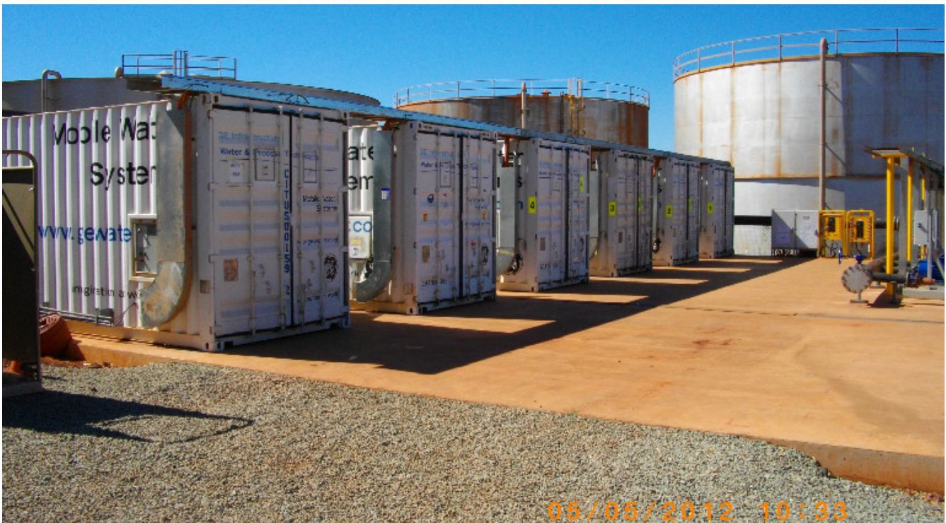
Photograph 4: Mobile RO Containers On Site
