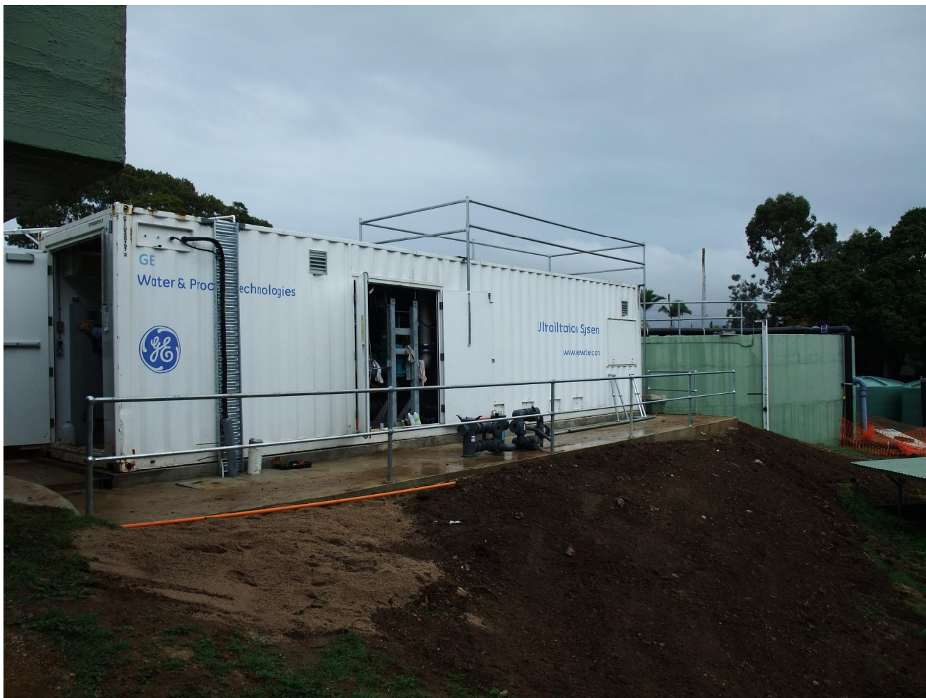
Photograph 5: Mobile UF Container on Site
