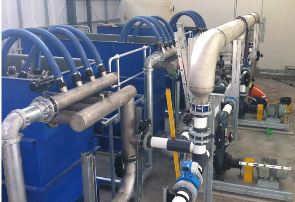
Photograph 1: Submerged Membrane Cells
