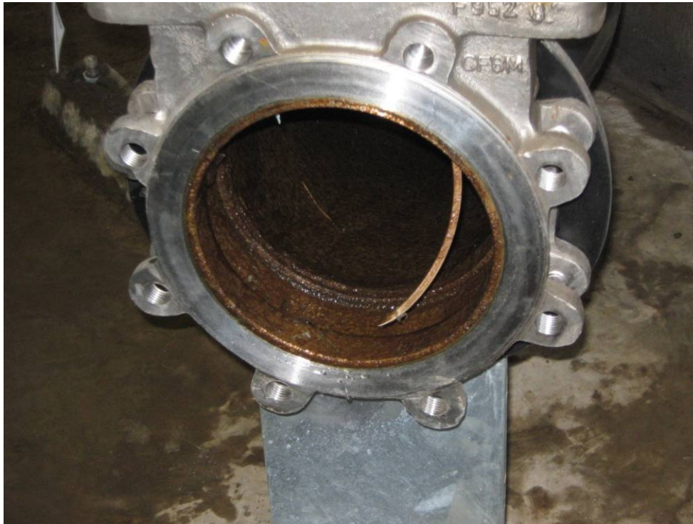
Photograph 8: Loose and broken valve seal Pump 3
