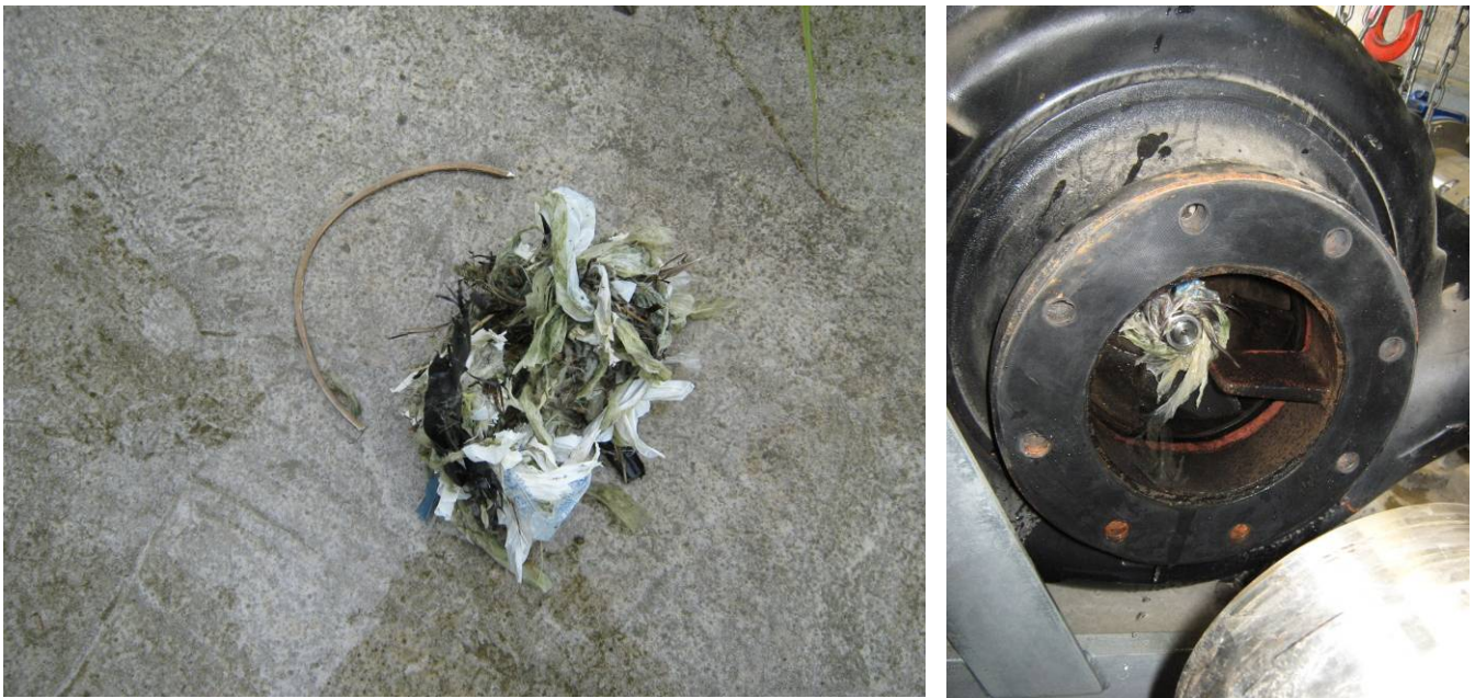
Photograph 3: Debris including part of a valve seal removed from the impeller of Pump 1
