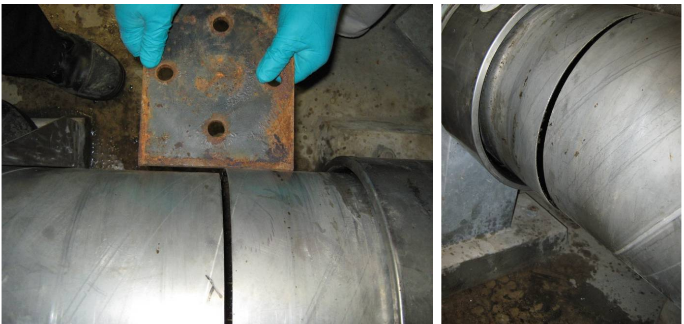
Photograph 7: Lateral and angular misalignment at Straub coupler in 300dia header pipe
