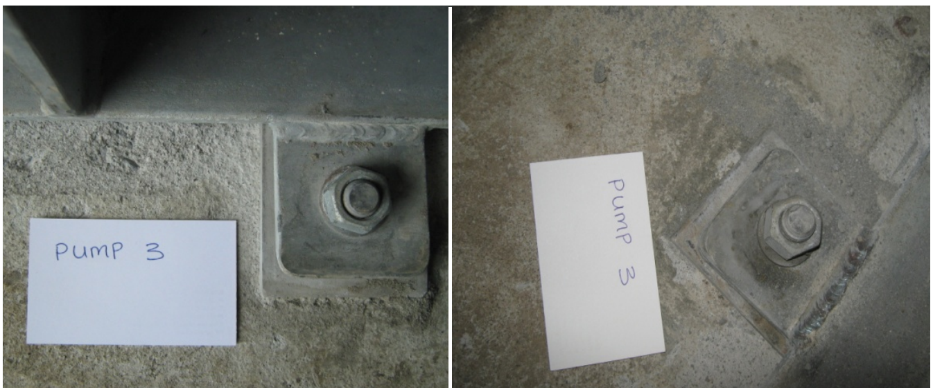
Photograph 10: Different size HD bolts Pump 3
