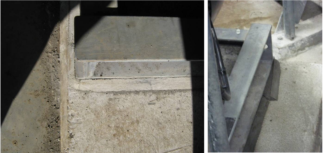
Photograph 1: Loose and cracked dry-pack at Pumps 1 and 2 motor ends
