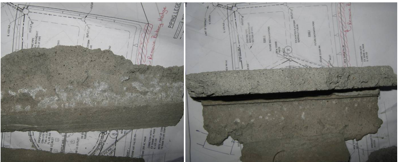
Photograph 17: Sample of original dry pack from under pump 2 plan view and edge view
