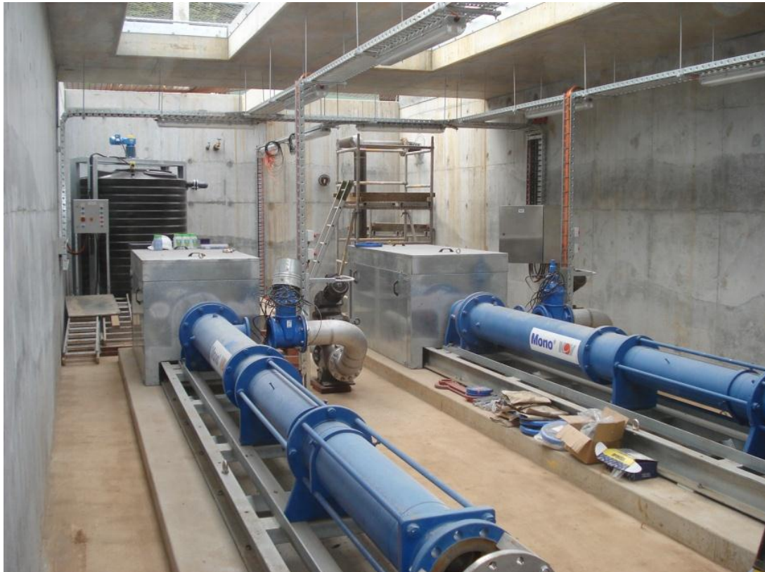
Photograph 1: The Flinders Sewage SPS chamber (During Construction) showing progressive cavity pumps
