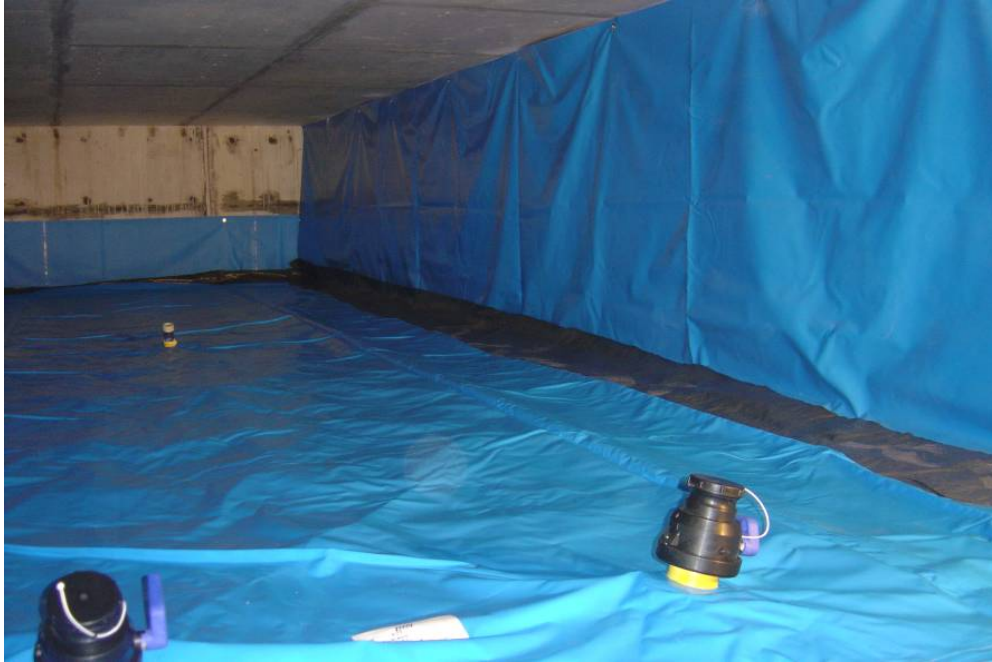
Figure 4: Flexible bladder tank laid out in utilities building basement
