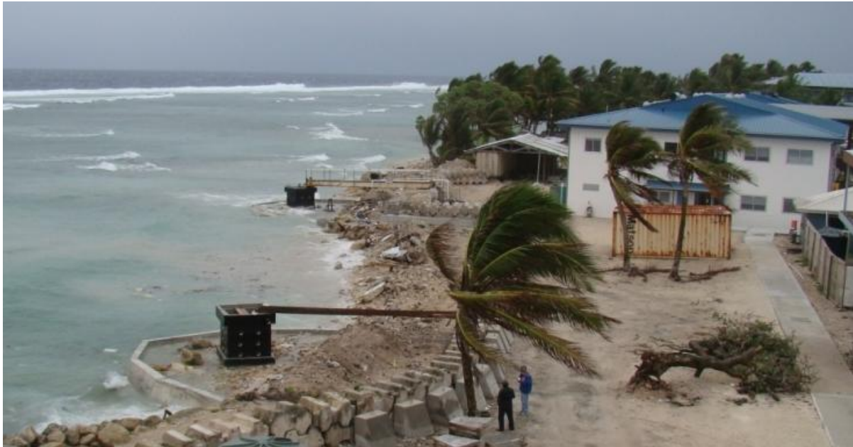
Figure 10: Sea wall structures – designed to resist ocean wave impact
