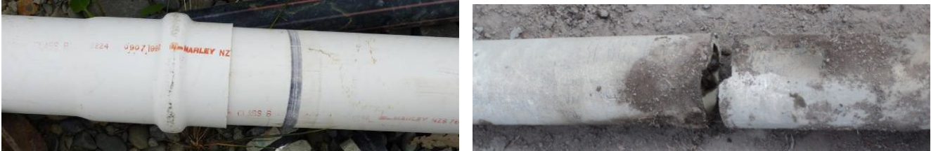
Photograph 2: Pipe Failures – Joint Pull-Out and Pipe Break
