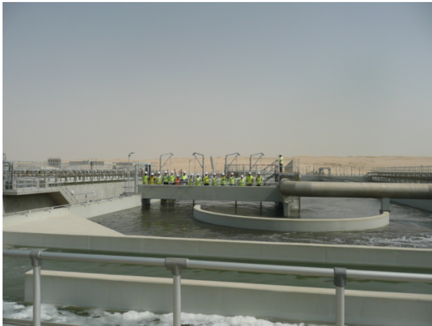
Figure 2 Wathba 2 WWTP BOOT Project during commissioning (taken when the first wastewater flow was received at the Wastewater Treatment Plant)
