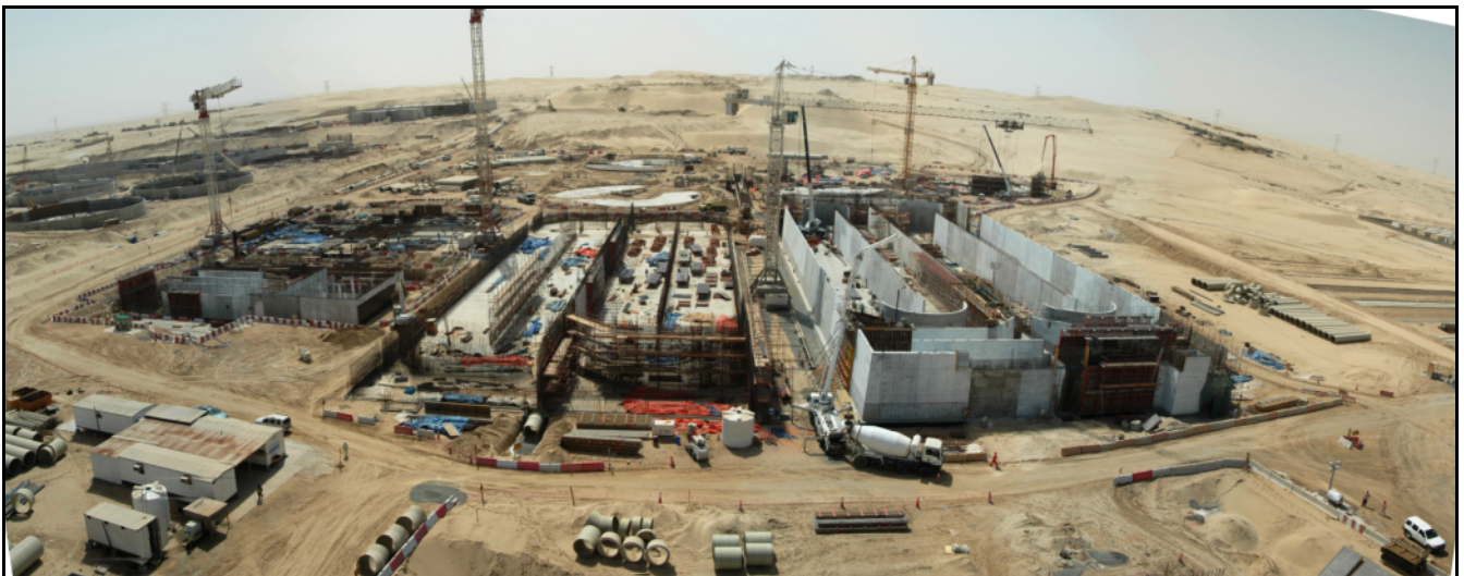
Figure 1 Wathba 2 WWTP BOOT Project in the early stages of construction (Photo taken from a tower crane)
