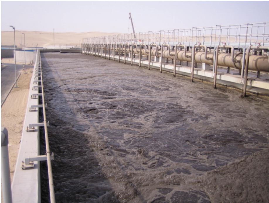
Figure 12 Wathba 2 WWTP Operation
