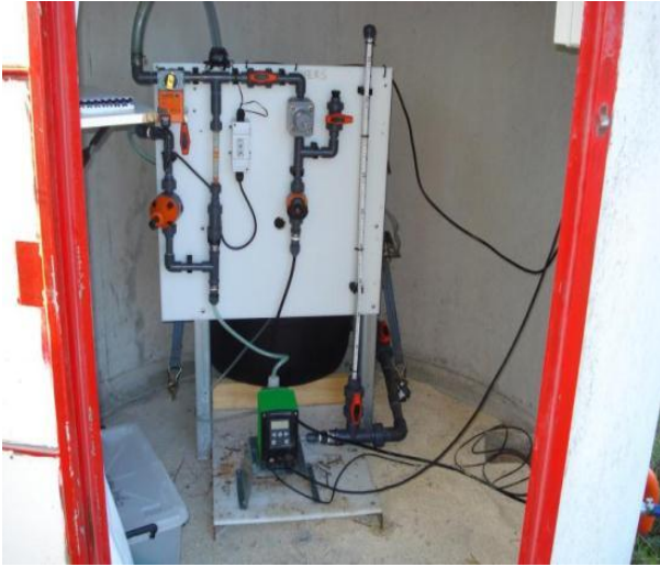
Dosing station installed in concrete container
