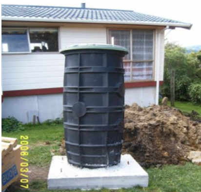
Photograph 1: Typical pump station unit prior to in-ground installation
