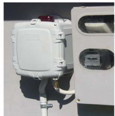
Photograph 3: Typical new house electrical connection
