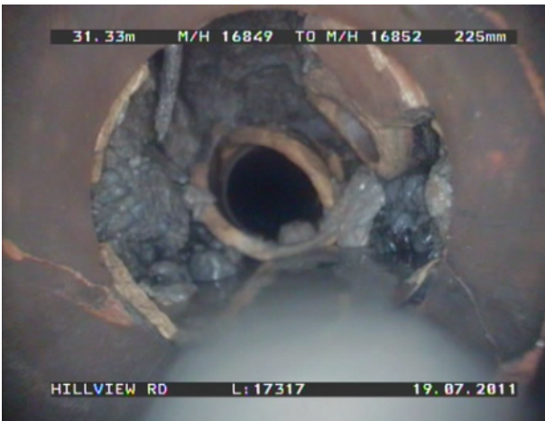
Photograph 3: "Example of the pipe damage"
