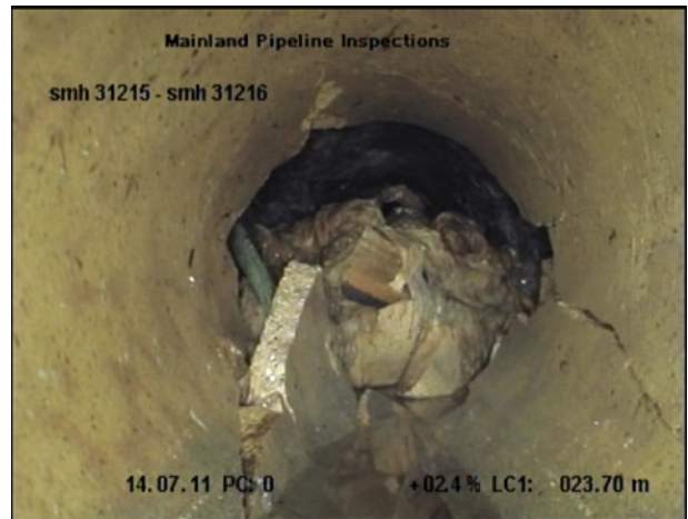
Photograph 4: "Example of the pipe damage"
