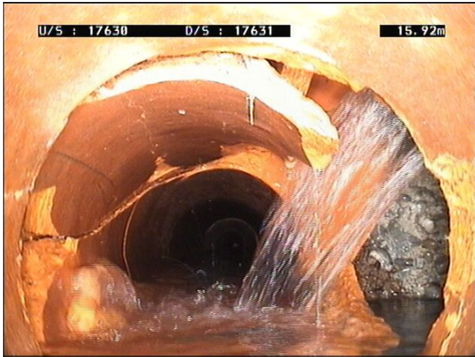
Figure 3: Breaks in EW pipe resulting in Tomo
