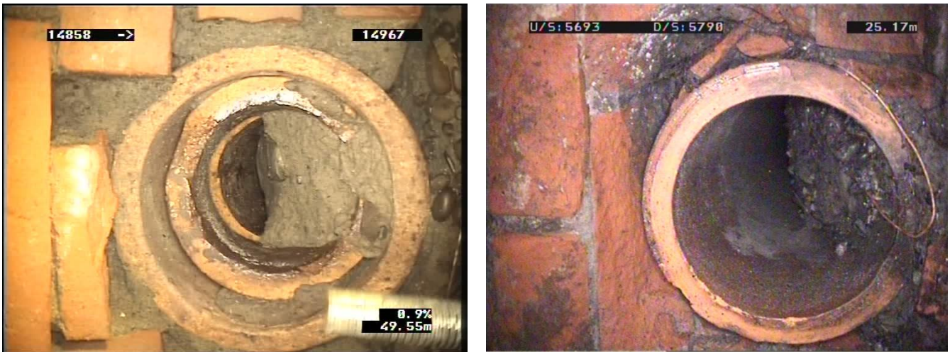
Figure 10 Silt infiltration via laterals
