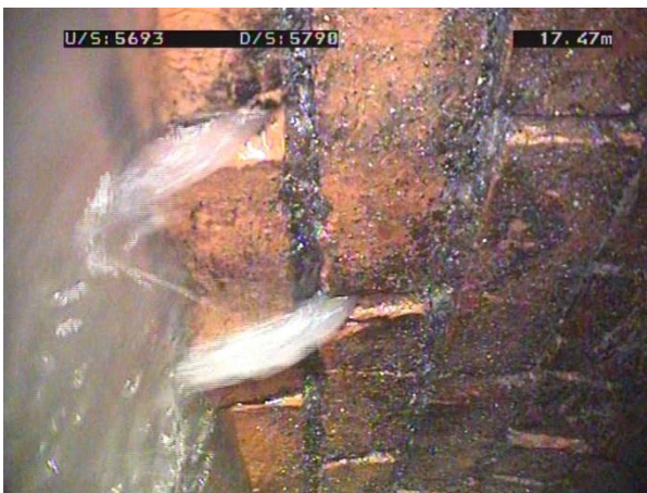
Figure 8 - Silt infiltration via defective brickwork
