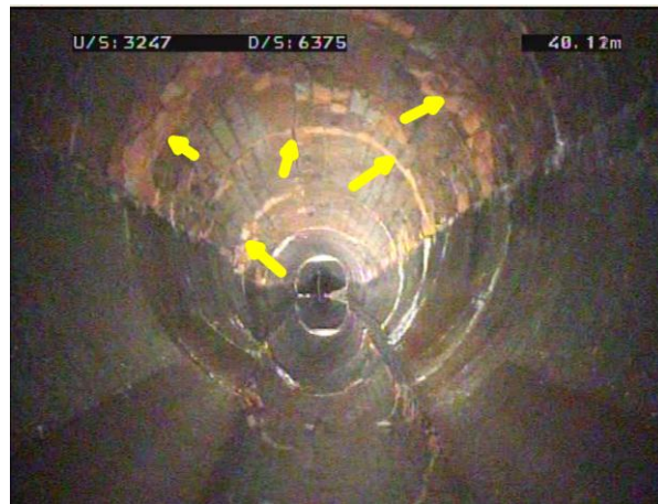
Figure 7- Circumferential & longitudinal cracking
