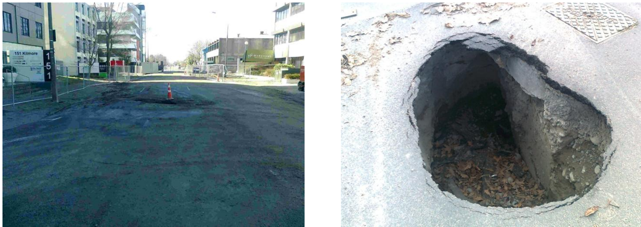
Figure 14 Kilmore St sinkhole (photo- Christchurch CC)
