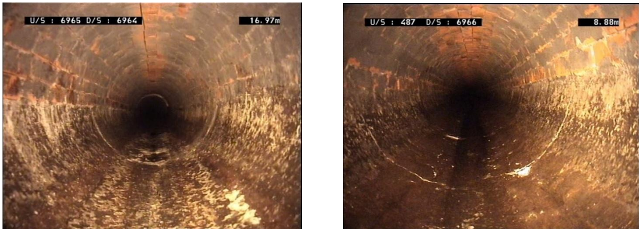
Figure 13 Deformed profiles in storm water brick barrels
