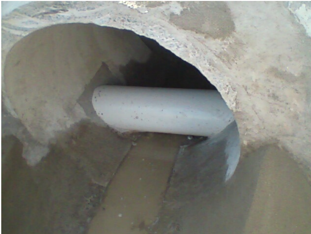
Photograph 2: Wastewater pipe through stormwater pipe
