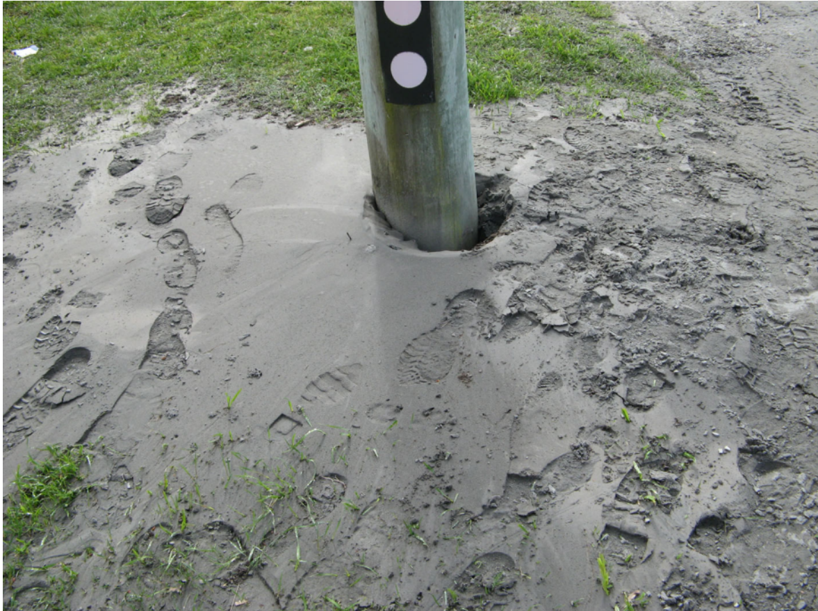
Photograph 4: Silt ejected around power poles
