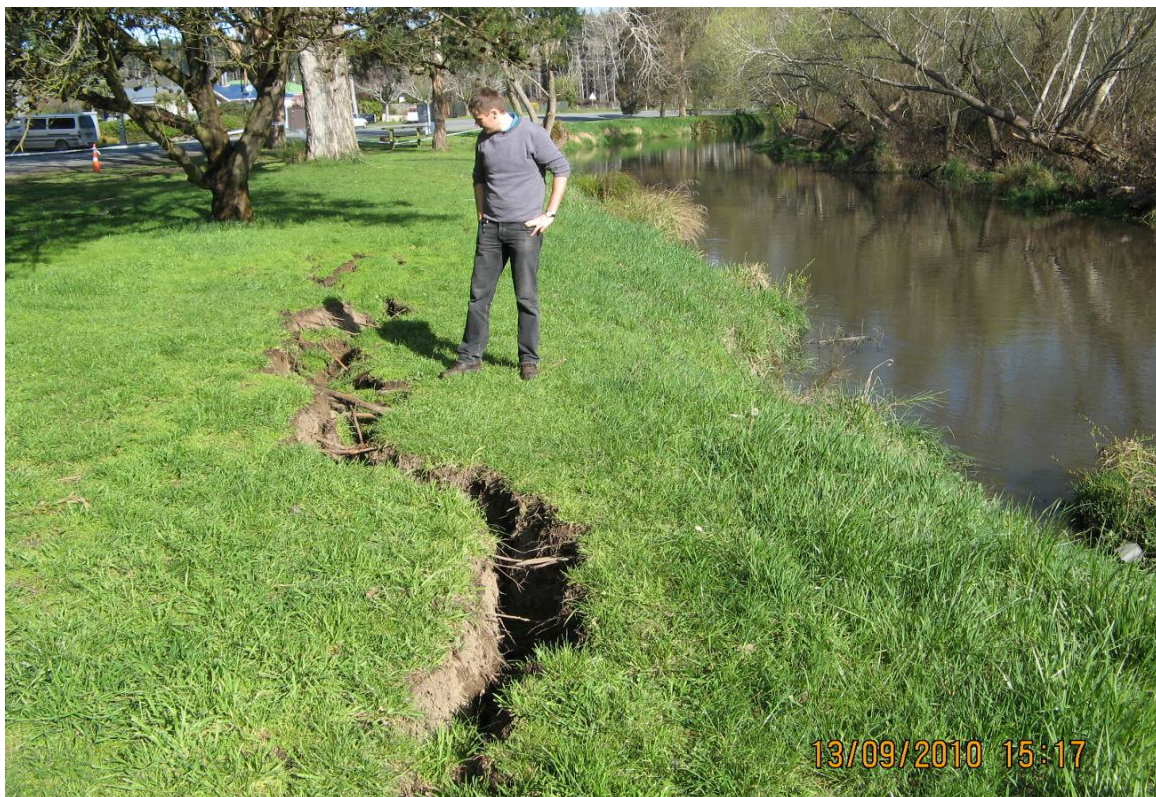
Photograph 1: Lower Styx Bank Slumping
