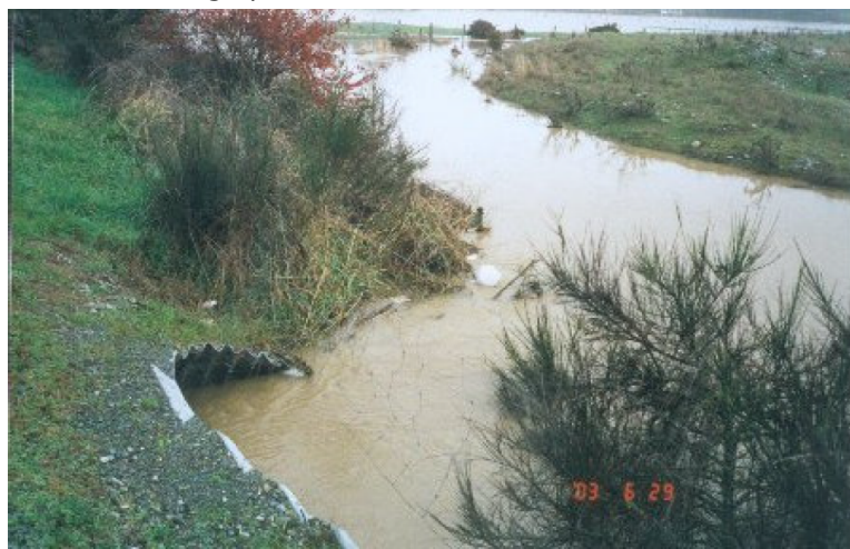
Photograph 3: Armco Culvert under Stafford Drive in flood – June 2003
