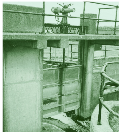
Figure 5: An example of a motor mounted, actuated penstock in a wastewater treatment plant
