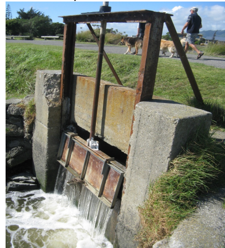
Figure 1: The existing level control weir on the Waimanu Lagoon outfall is a manually operated penstock that can be wound upwards to increase discharge through the 1800mm diameter pipe.
