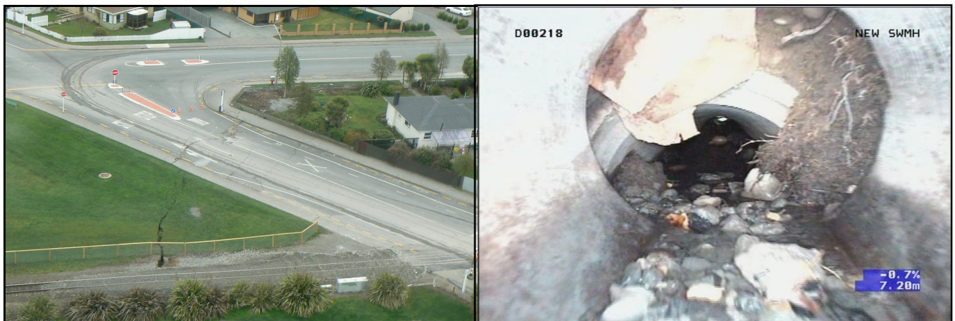
Photographs 4 & 5: Damage at extent of lateral spread on Peraki Street. Cracking in road and reserve is evident next to stormwater manhole (left). Damage to 450mm pipe.
