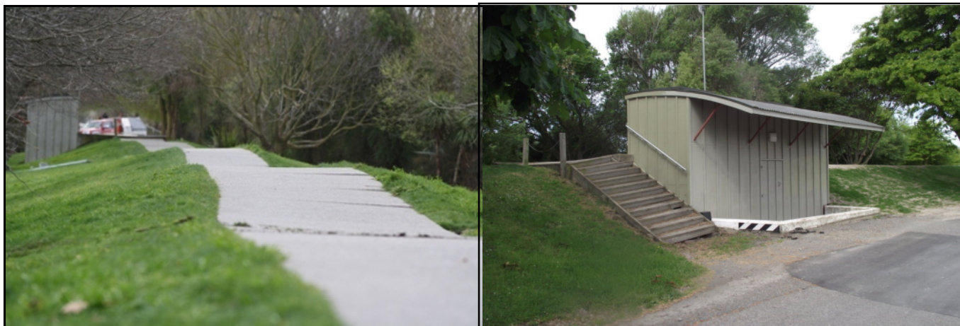
Photographs 6 & 7: Laterals spread of stop bank adjacent Dudley Pump Station.
