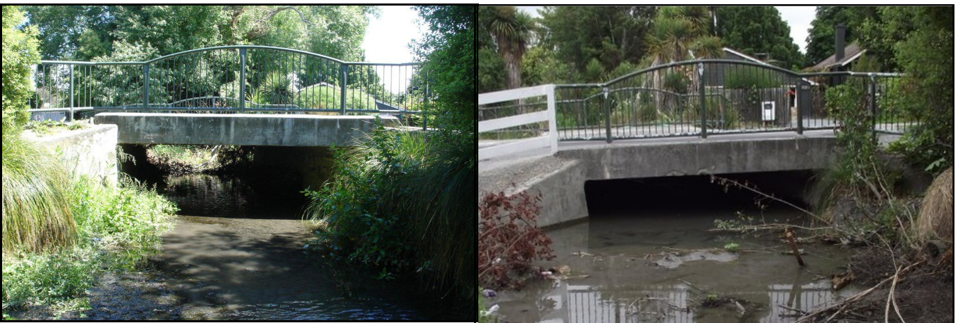
Photographs 2 & 3– Hilton Street Culvert (downstream view), pre-earthquake (left) water level approximately 1100mm below soffit and post-earthquake (right) water level approximately 600mm below soffit
