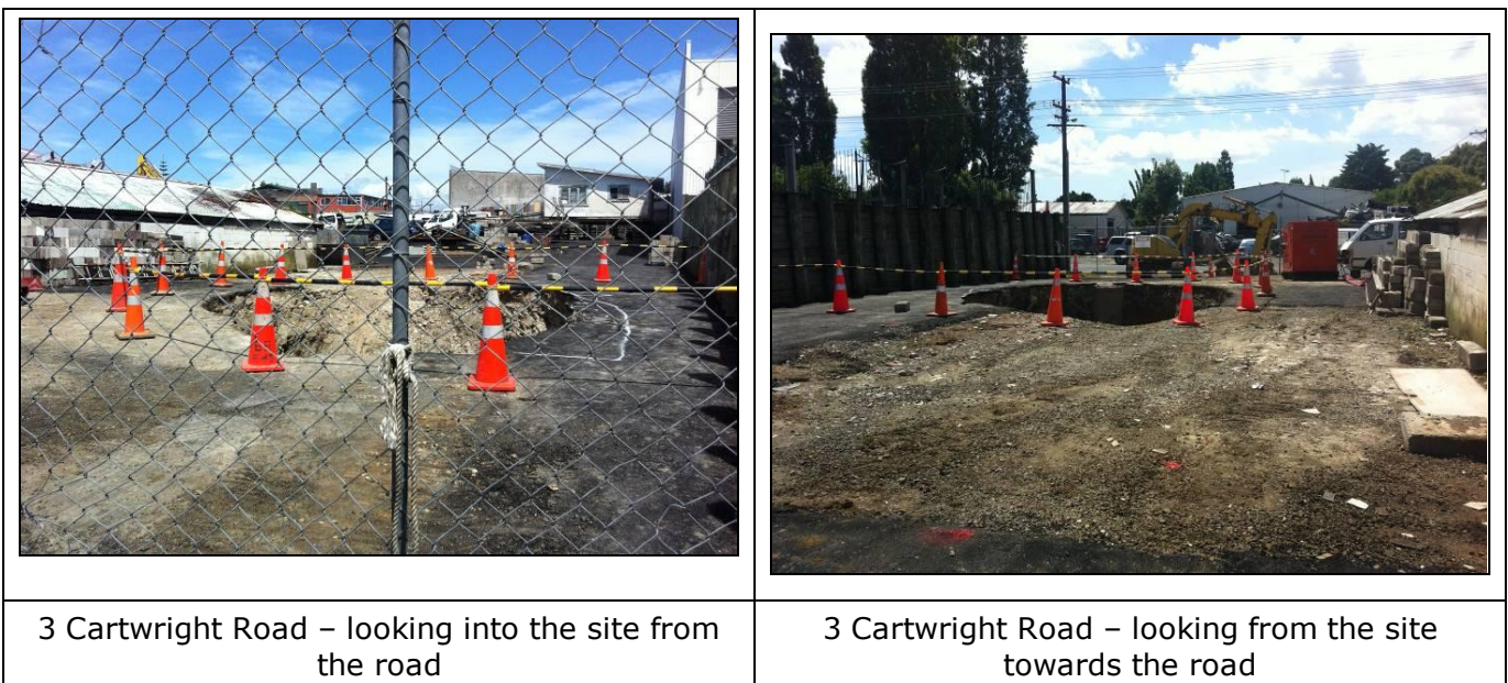
Photograph 1: Sinkhole formed within 3 Cartwright Road
