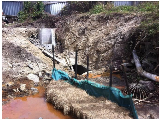
Photograph 3: Clearance of overland flow path and relief points cut into SW network
