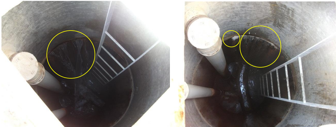
A: Manhole before leak repair (circle)
