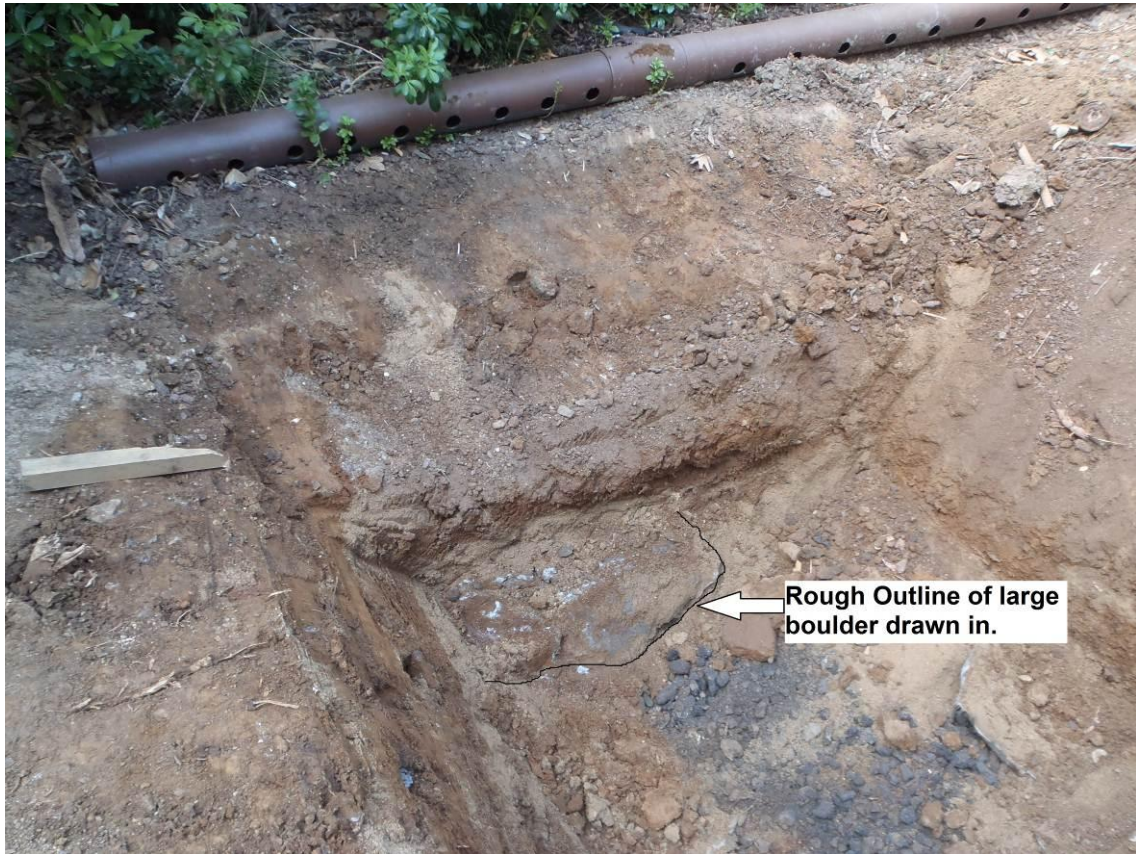
Photograph 3: Large boulder in original media bed
