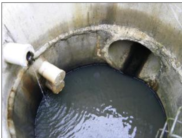
Photograph 57: Showing Drain Valves
