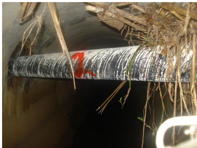
Figure 5 A large water supply pipe running through the big twin culverts
