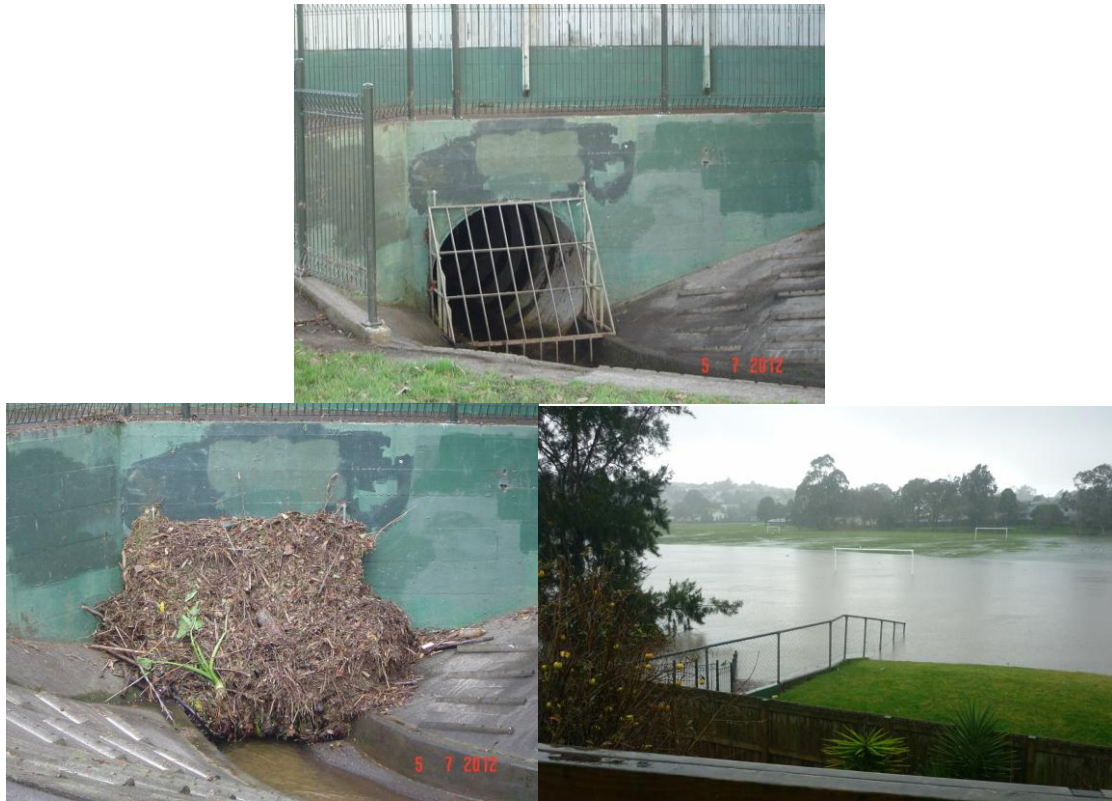
Figure 6 A totally blocked 1.8 m diameter inlet and the flooded, large recreational reserve resulting from that blockage
