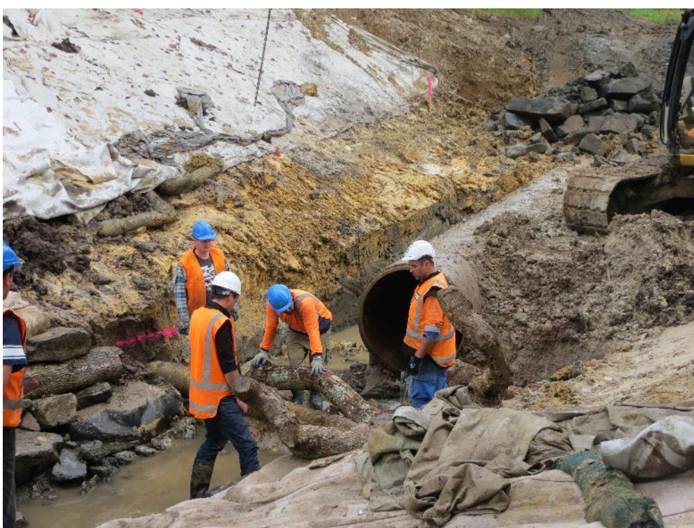
Figure 7: The design and construction team working through sections of the Avondale Stream
