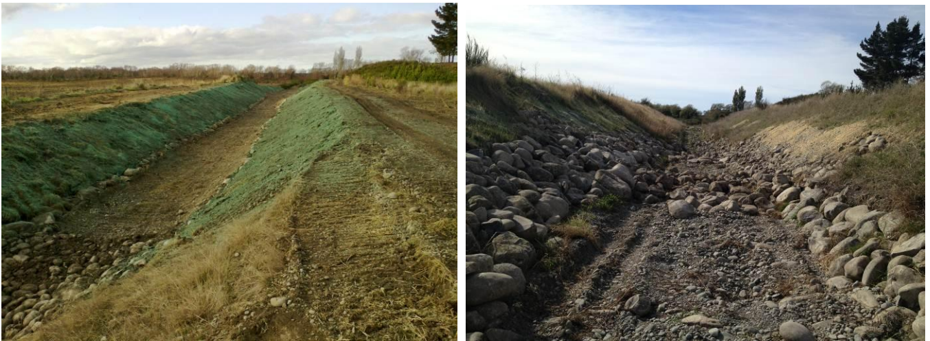
Photographs 5, 6: Completed Wheatstone Drain bank stabilisation works before and after installation of rock sills
