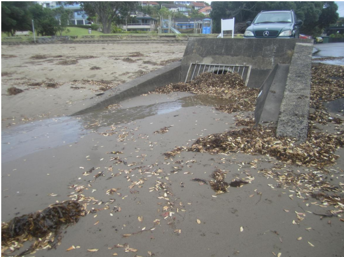
Figure 5 A 1.5 m diameter beach outlet which was blocked by sand and debris after Cyclone Lusi passed Auckland
