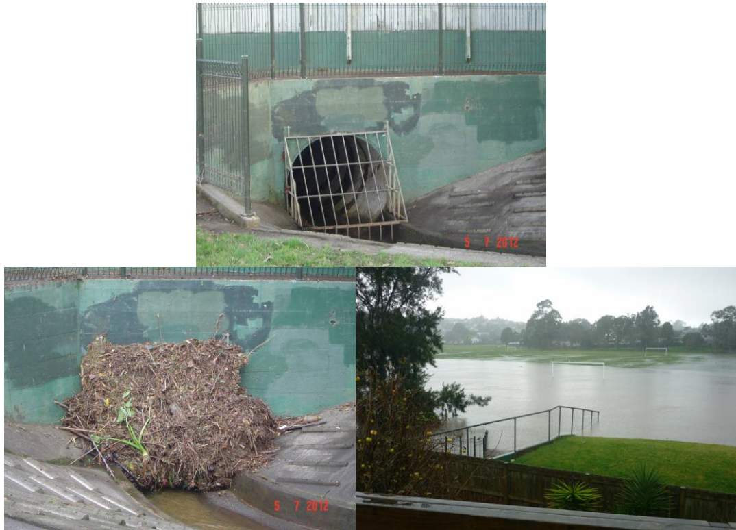
Figure 2 A totally blocked 1.8 m diameter inlet and the flooded, large recreational reserve resulting from that blockage (Source: Tian et al, 2013)
