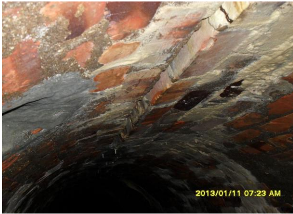
Fig. 6 Displaced brick, longitudinal crack at crown
