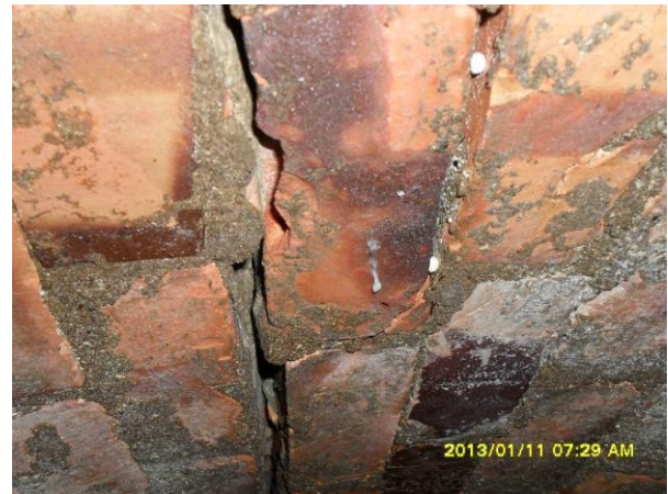
Fig. 9 Multiple cracking, old repointing
