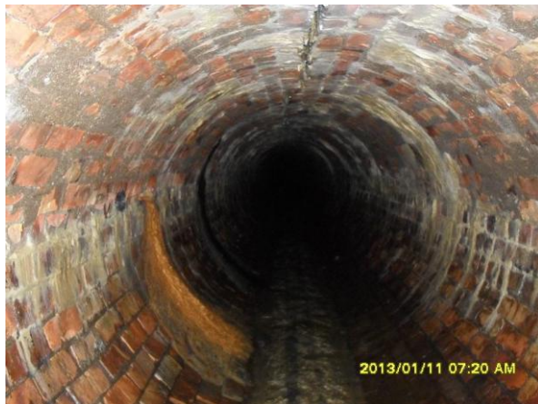
Fig. 8 Extended longitudinal crack, deformation
