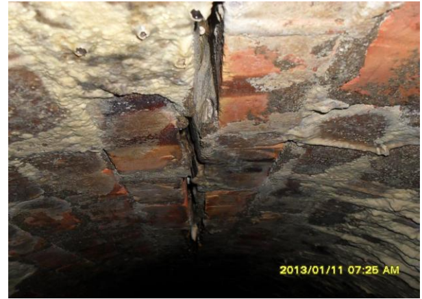
Fig. 7 Extended longitudinal crack, lime deposits
