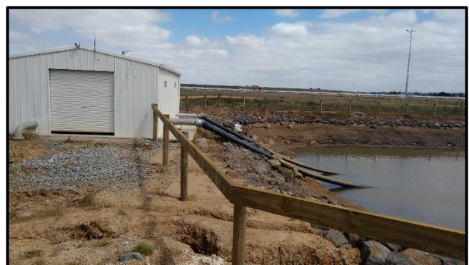
Figure 2-11: Irrigation Dam Outlet Pump
