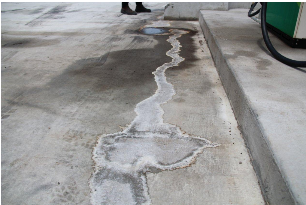
Photograph 1. Dried DEF on a forecourt.
