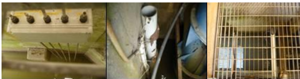
Photograph 5 Pump controls – electric probes and ultrasonic level control
