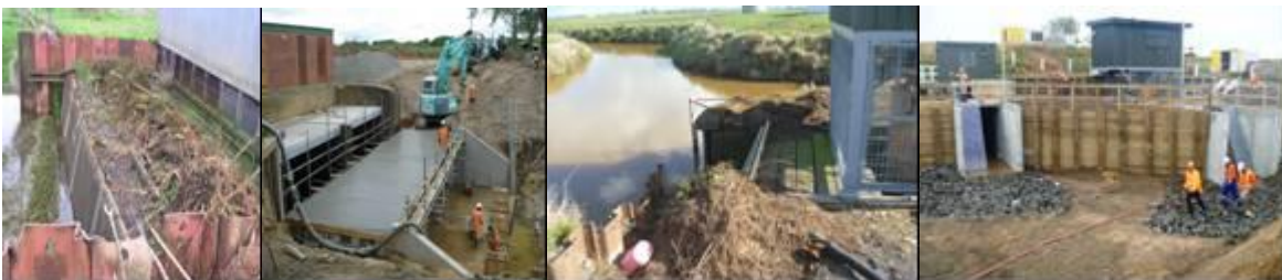
Photograph 1 Old and upgraded inlet bays, screens and platforms
