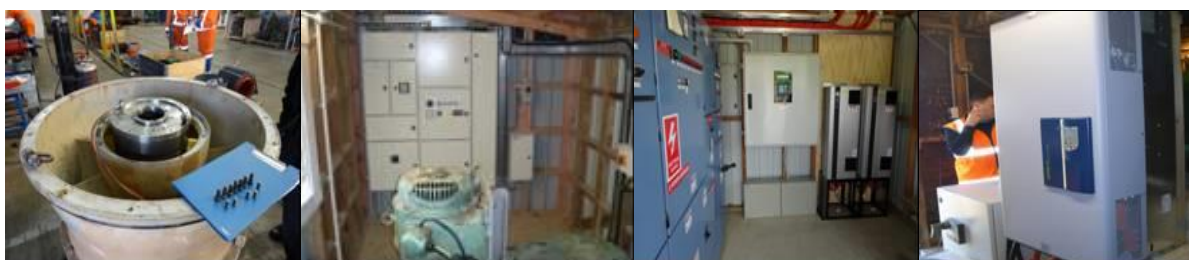
Photograph 6 Soft starters and variable speed drives
