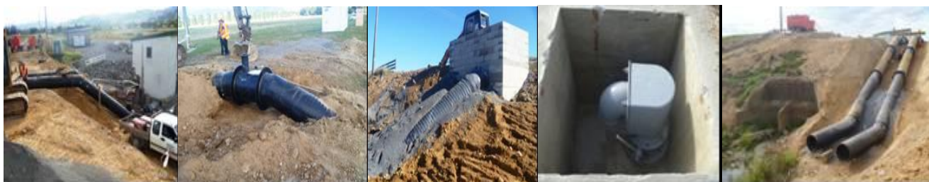
Photograph 7 HDPE siphon pipe outlet with a siphon breaker at the top of stopbank
