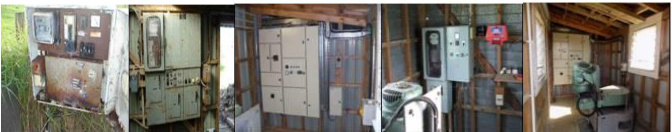
Photograph 4 Old and newly installed switchboards
