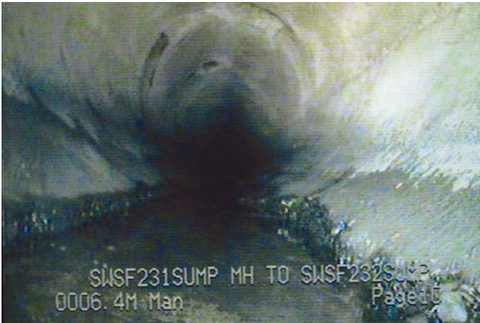
Photograph 9: CCTV Image of Queen Street 900mm Diameter Main
