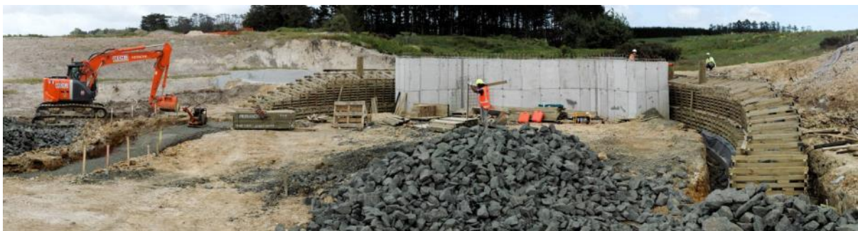
Figure 8. A stormwater outfall structure under construction – upon completion it is hidden behind the crib wall.
