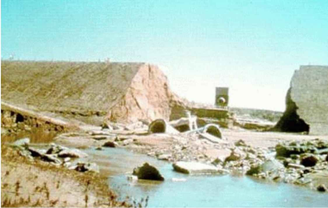
Example of dam failure at conduit
