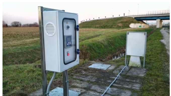
Figure 15: monitoring station along Passante di Mestre
