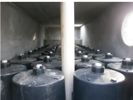
Figure 11: filtrating cartridges inside a treatment plant
