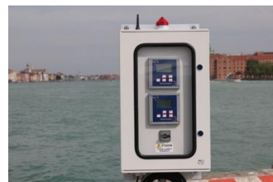
Figure 4: view of the control panel in an outside configuration
