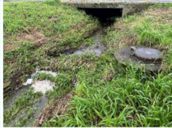
Vegetation/sediment/debris built-up in the waterway restricting flow, grass needs mowing, potential contaminants in the water
