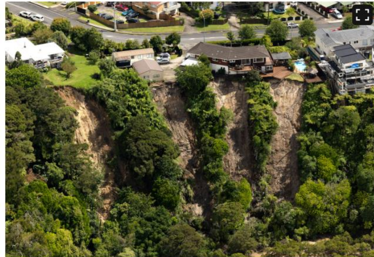
Hanging on the edge - landslides threaten homes on Colwill Road, Massey. Photo / Brett Phibbs
