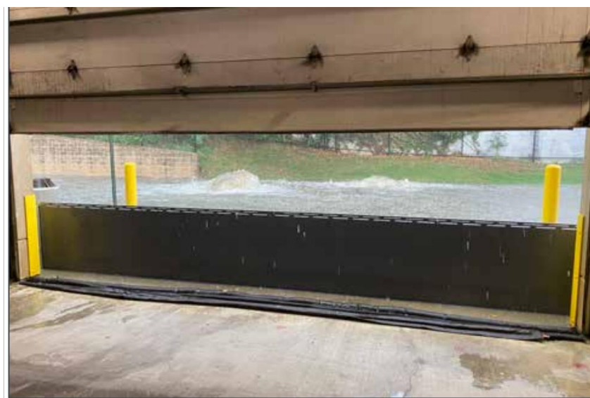
Passive flood gate at entrance to parking garage
