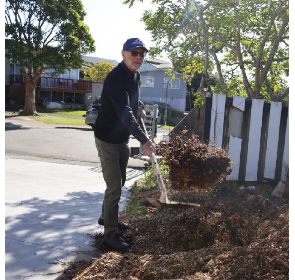
Mayor Wayne Brown shovelling bark from blocked manhole.
