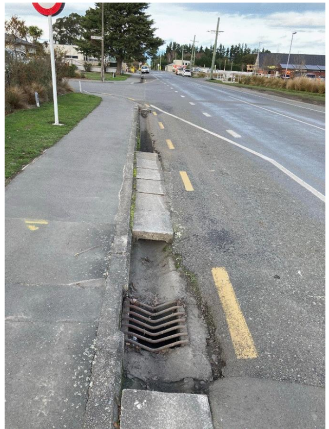
Plate 14: Pit and pipe network with deepish kerb and channel on Weedons Ross Road
