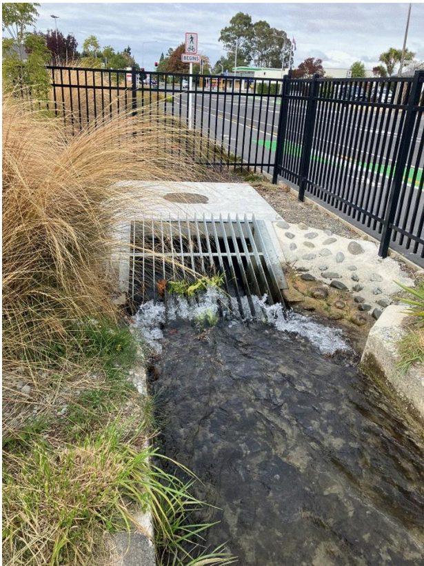
Plate 17: Piped stock water network inlet on Weedons Ross Road
