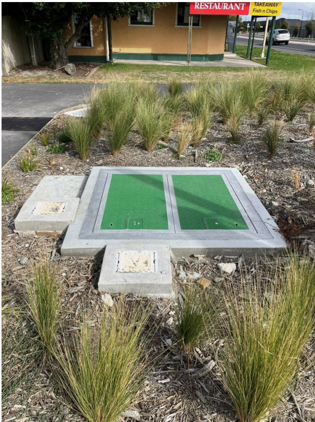
Plate 21: Flow splitter chamber at SH73/Weedons Ross intersection
