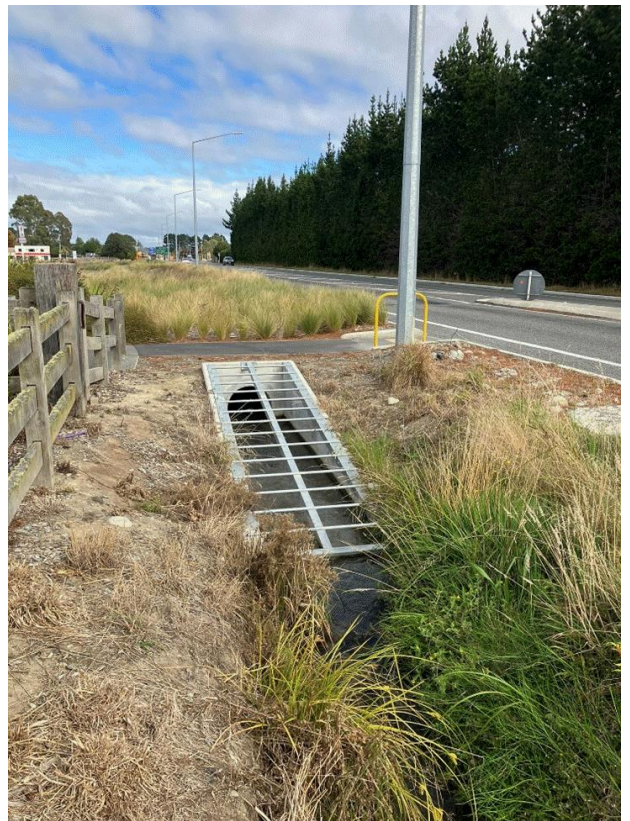
Plate 20: Mountable headwall on SH73
