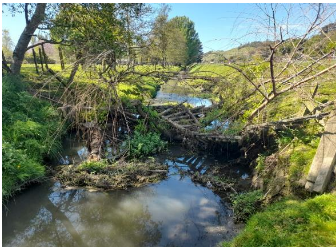
Figure 5: Partial blockage in Waipukurau drainage channel
